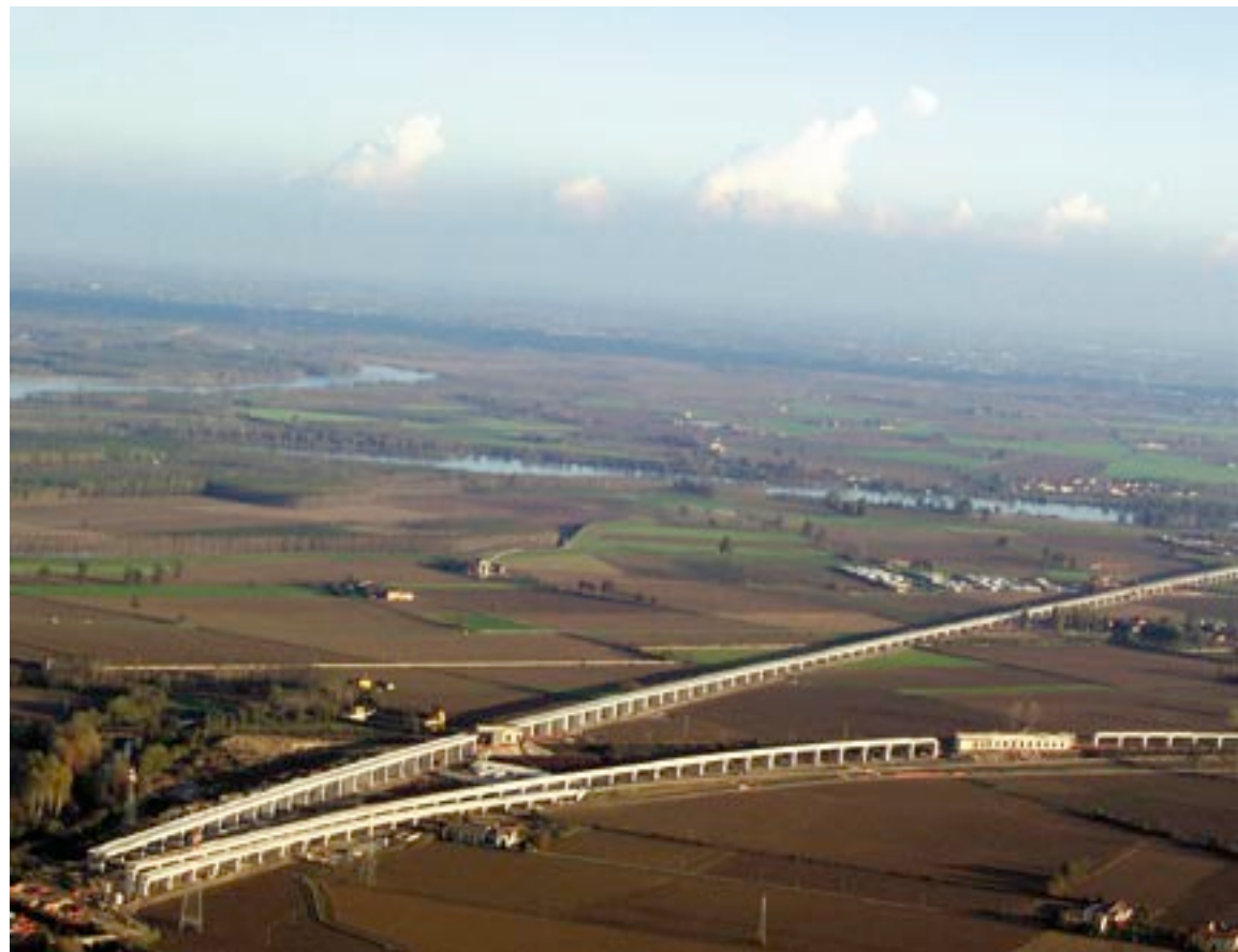
Construction of the new high-speed Milan to Bologna rail connection, carried out by Italferr and other companies and contractors of FS, the Italian state railway, is managed in accordance with an ISO 14001-based EMS.
