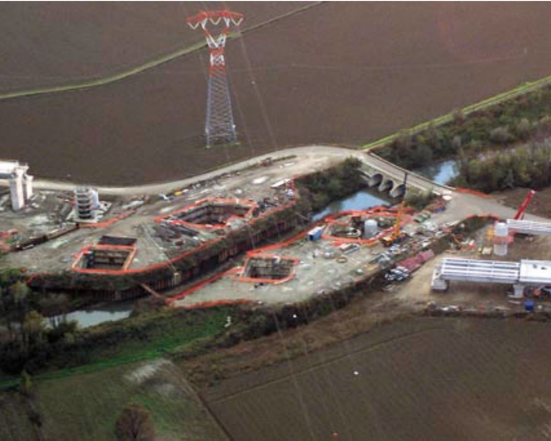
Another view of the construction of the new high-speed Milan to Bologna rail connection.
